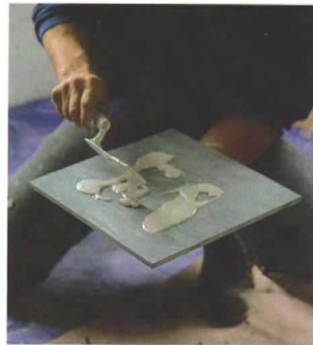
Epoxy seals the backs of the green-marble tiles. Green marble reacts badly to water-based adhesives, so the backs of the tiles are sealed with nonporous epoxy. A trowel spreads the thick and gooey epoxy.
